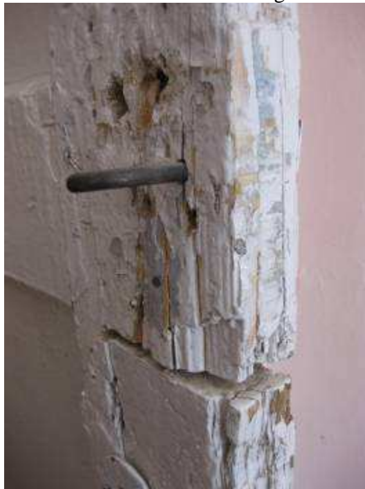
Doors needs to be changed
