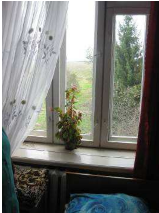
Windows need to be replaced in the third floor
