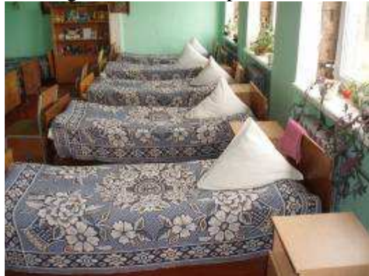
Windows have to be repaired inside in the sleeping rooms
