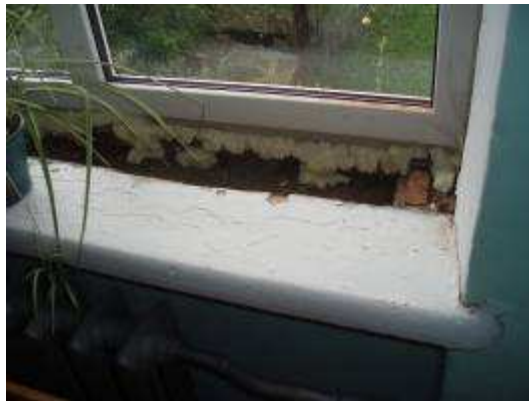
Inside nothing was done to adapt to the new windows
