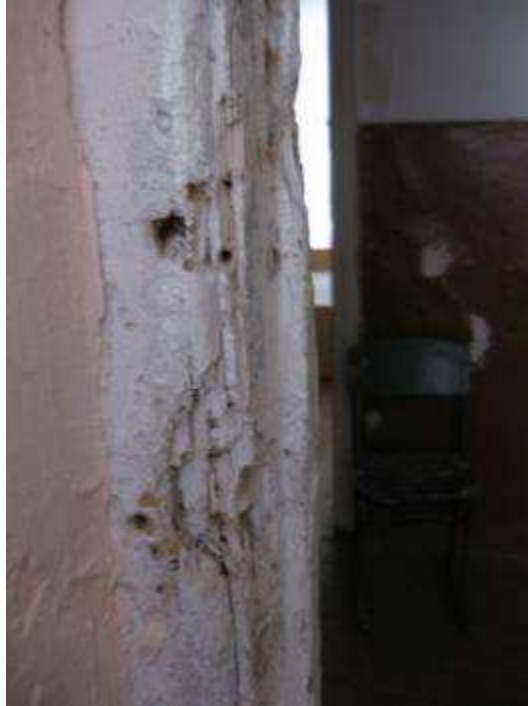
Doors needs to be changed
